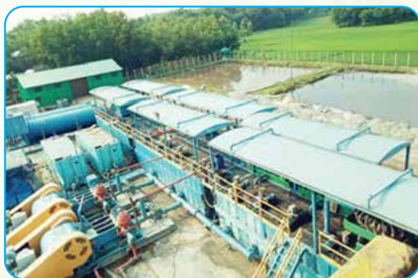
Mud Circulation System of Rig
