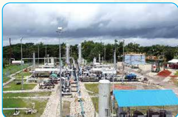
Glycol type Gas Process Plant at Shahbazpur Gas Field
