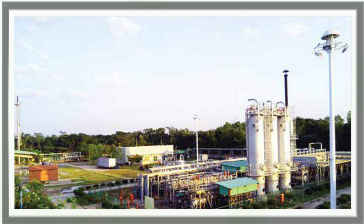
Process Plant of Srikail Gas Field
